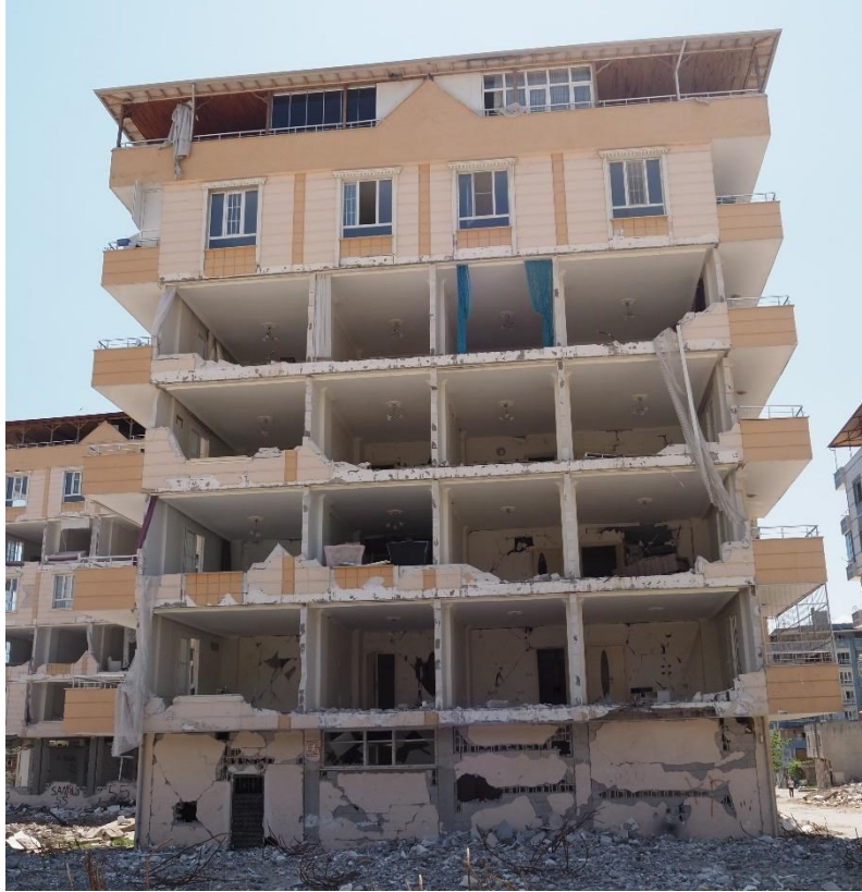
Figure 5.4.10 Overturning of infill walls, because of out-of-plane loading.
