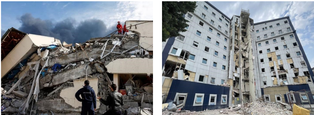
Figure 5.5.9 (a) Collapse of the Iskenderun State Hospital (credits: REUTERS/Tessier) (b) partial collapse of a private hospital in Antakya (Credits: Sumer et al.)
