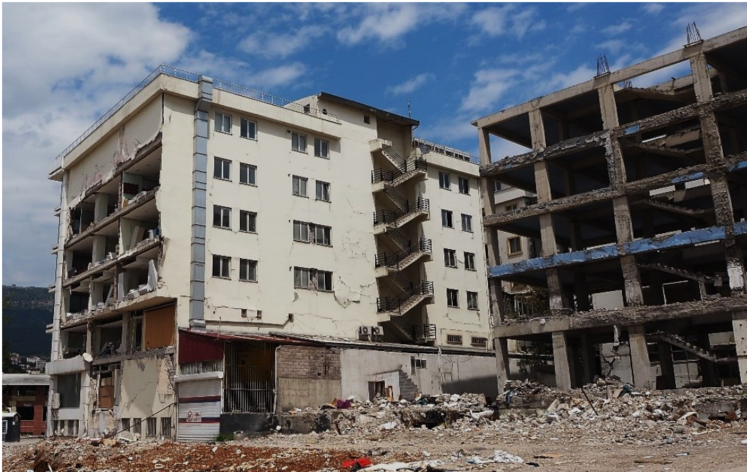
Figure 5.4.11 Infill walls with diagonal cracking, along the direction of the earthquake and failing to out-of-plane loading, perpendicular to the main direction of the earthquake.
