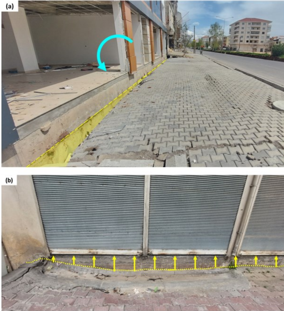
Figure 3.32 a), (b): Cases of permanent tilting of buildings in Gölbaşı city, due to rocking oscillation that results in uplifting displacements in the front side of the structures (37.788762N, 37.649529E).
