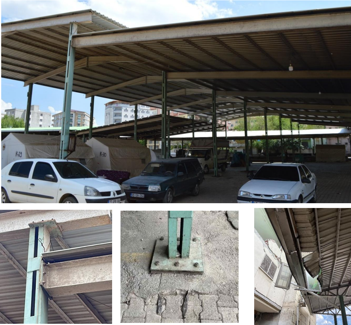
Figure 5.2.2 Roof structure of outdoor parking in Islahiye, with structural details showing no significant damage from the earthquake other than the ones caused by an adjacent building.
