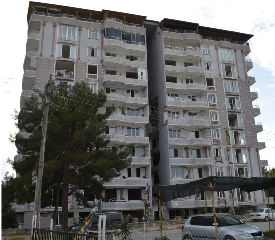
Figure 5.2.3 Top floor roof on a 10-story building in Adiyaman. Despite the damage to the main building and the increased top-floor acceleration, no significant damage can be observed.
