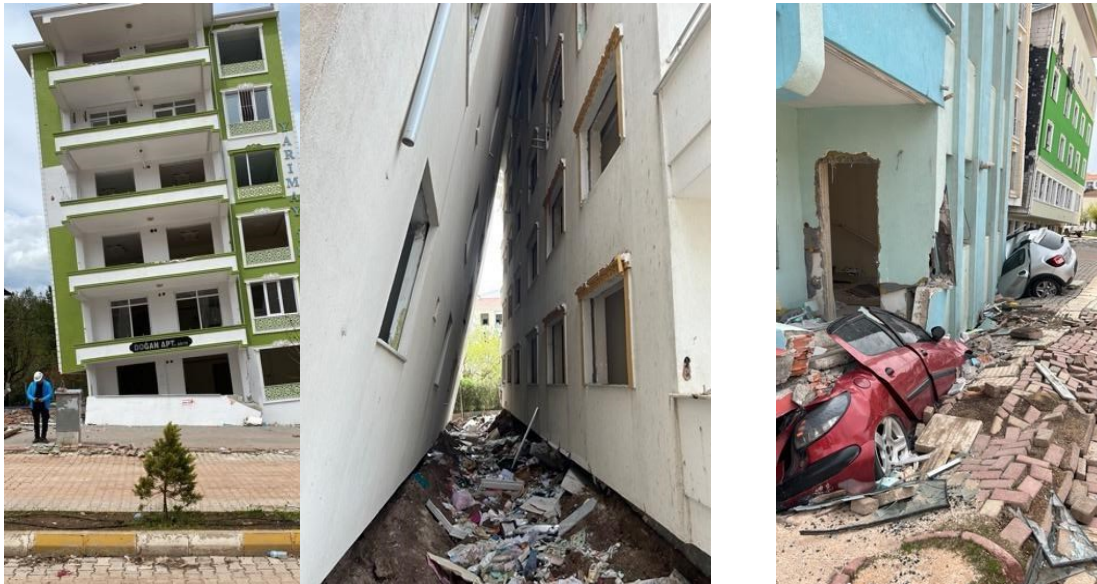
Figure 3.8 Zoning of extensive damage to buildings along and around recent lake and river deposits in a basin formed by two faults in the Gulbasi area.
