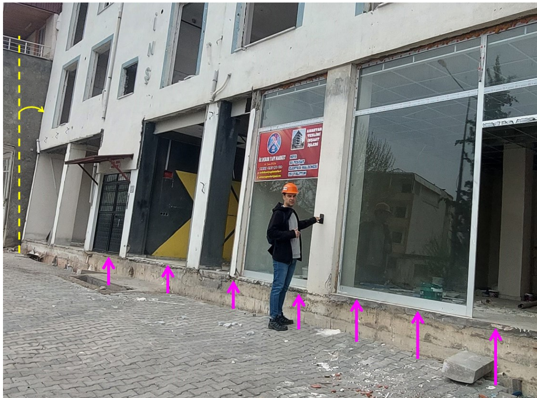
Figure 3.34 RC building with permanent tilting. Uplifting displacements in the façade (37.790129N, 37.651630E)
