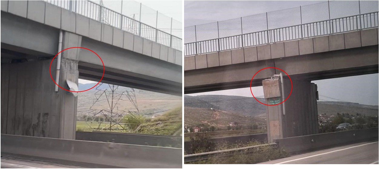
Figure 6.6 Shear key (stopper) failure of a seismically isolated bridge of Kahramanmaras interurban network
