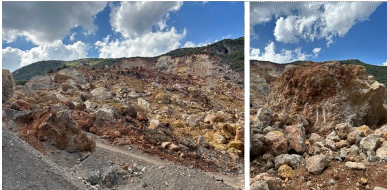
Figure 3.50 A rotational landslide in Tepehan village, Altınözü, Hatay (N36 9'39.3"; E36 13'17.9"). A clay-rich weathered limestone mass slide along the interbedded marl
