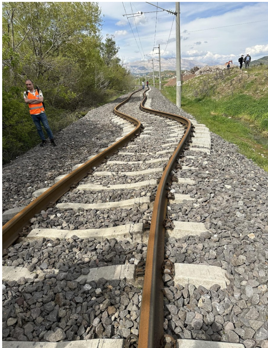
Figure 6.11 Railway track damage
