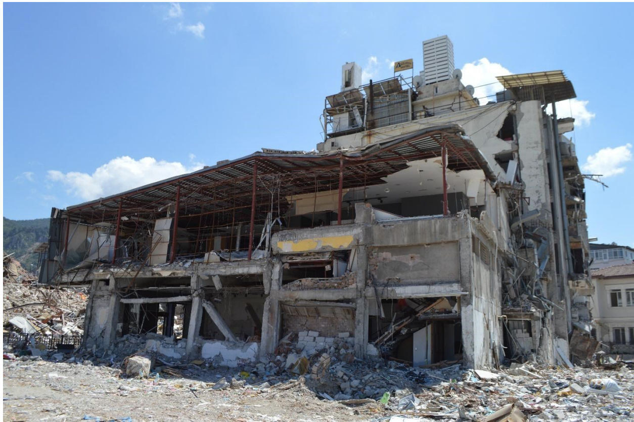
Figure 5.2.7 Top floor steel roof of a heavily damaged concrete building mainly due to pounding of the adjacent collapsed building (Antakya).
