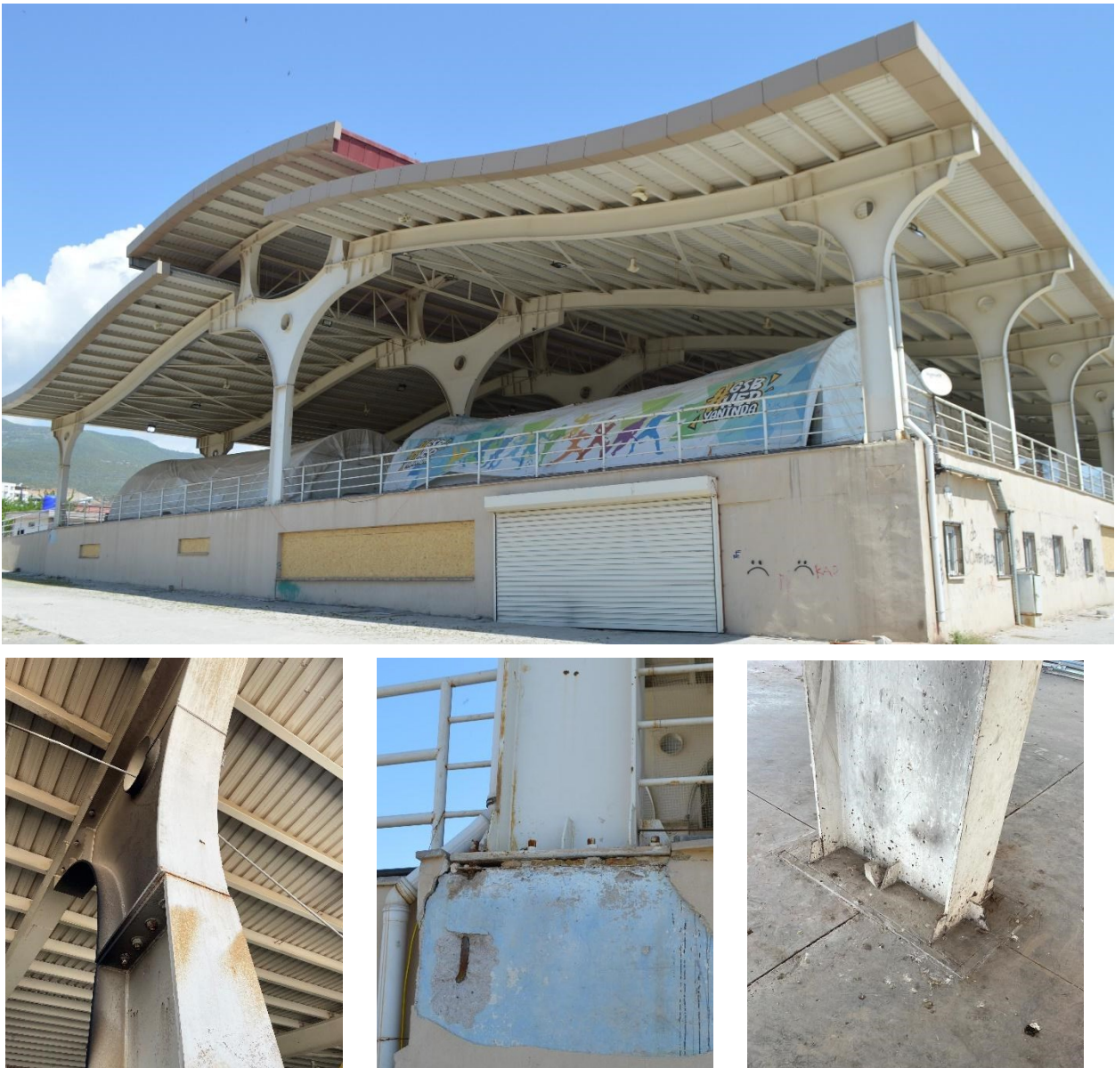
Figure 5.2.1 Roof structure of the municipal market in Nurdağı, with structural details showing no significant damage from the earthquake.
