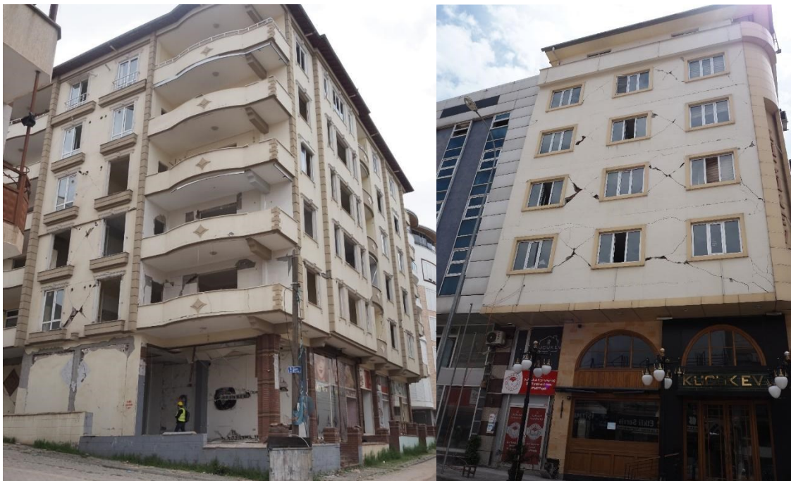
Figure 5.4.9 Extensive bi-diagonal cracking.
