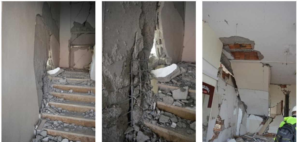
Figure 5.1.23 Damage to stairways and associated local damage to the vertical framing elements and asmolten slab-stairwell connection . Photo credit: C. Zeris (Adiyaman)
