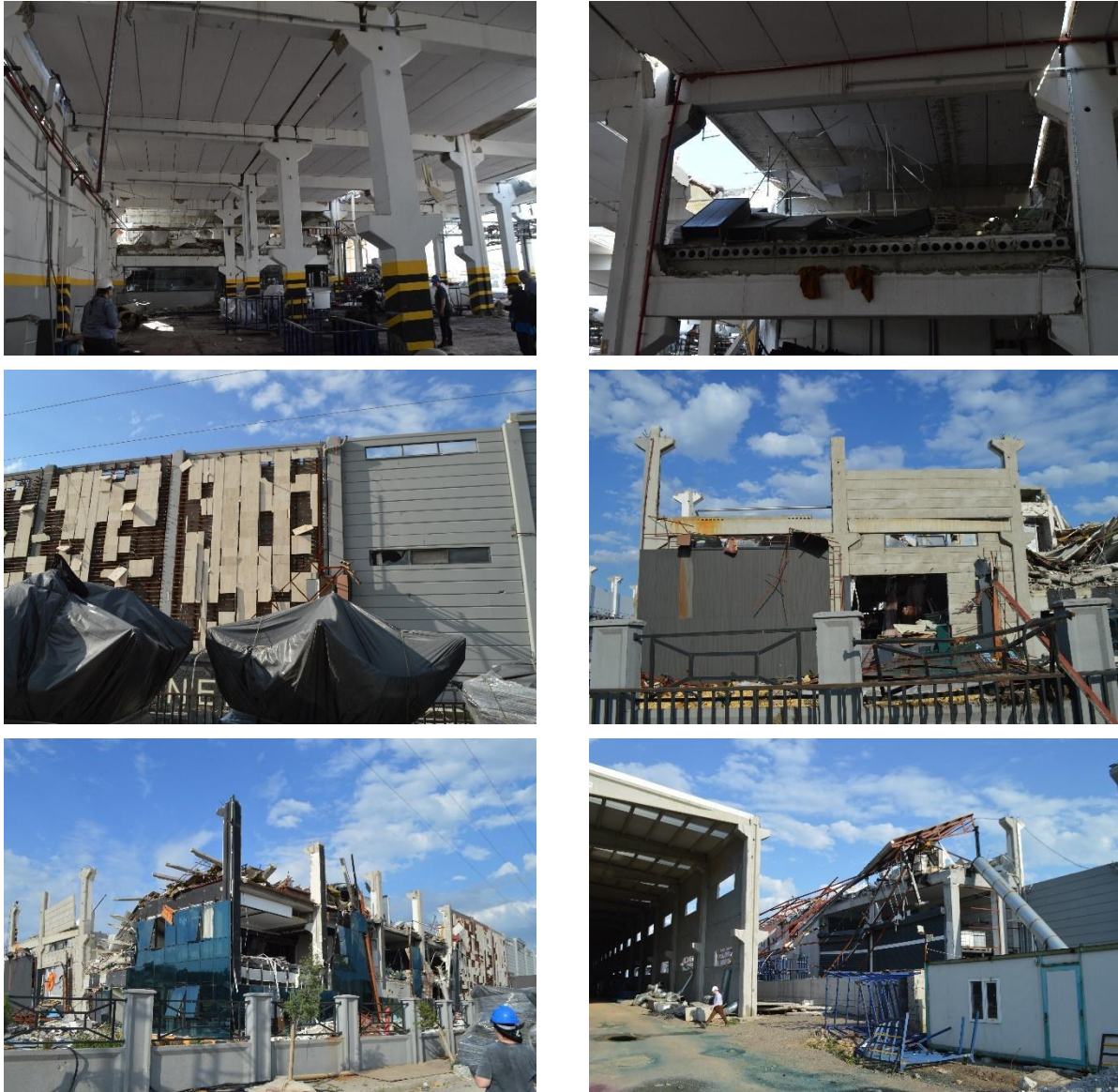
Figure 5.3.3 Various types of failures of reinforced concrete industrial buildings and their structural steel appendages (Kahramanmaraş).
