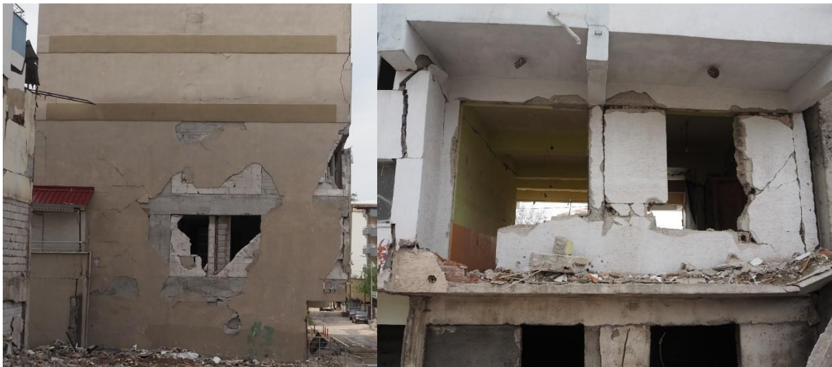
Figure 5.4.8 Separation of the infill wall from the frame and (partial) overturning.
