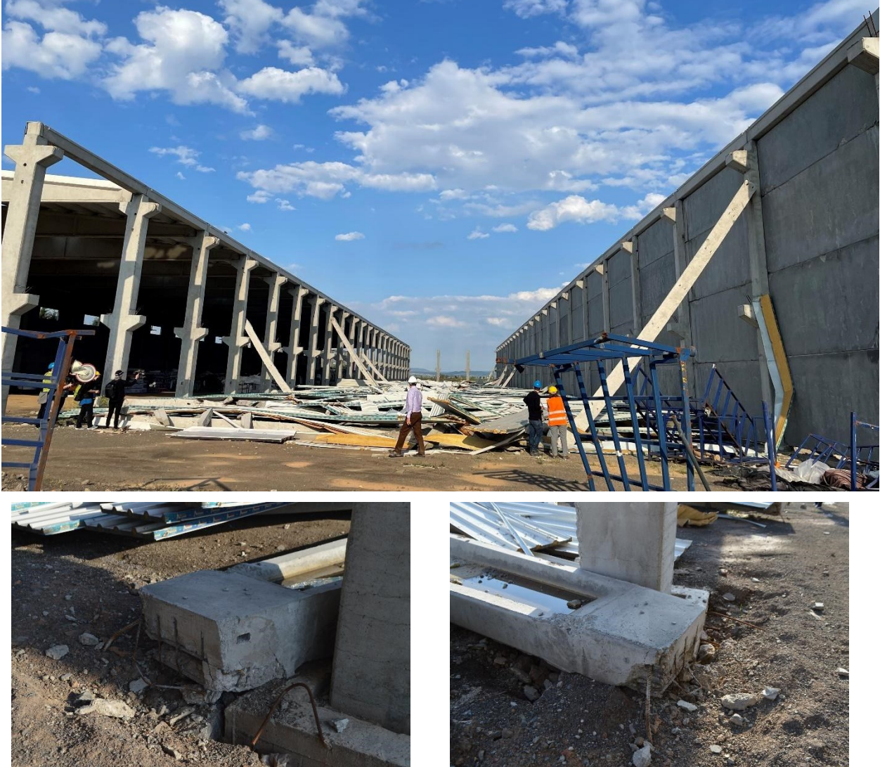
Figure 5.3.2 Total collapse of the middle bay of a reinforced concrete industrial building and details of the prestressed beam end (Kahramanmaraş).
