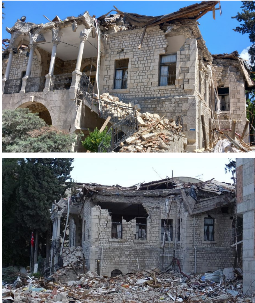
Figure 5.6.20 Antakya, collapse of the upper storey, as a result of the action of the RC slab (upper photo: A.Sextos)
