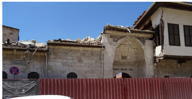
Figure 5.6.39 Damage observed in the standing parts of the Habib-i Neccar Camii
