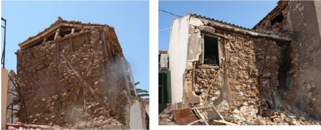
Figure 5.6.16 Vrissa, Lesvos Island, after the 2017 earthquake. The collapse of the exterior leaf of masonry revealed the interior timber-framed masonry (NTUA Report)
