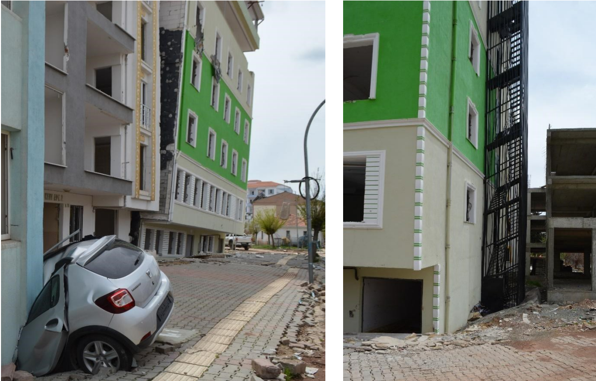
Figure 5.2.5 Fire escape staircase failure in Gölbaşı due to soil liquefaction and extreme settlement of the main building.
