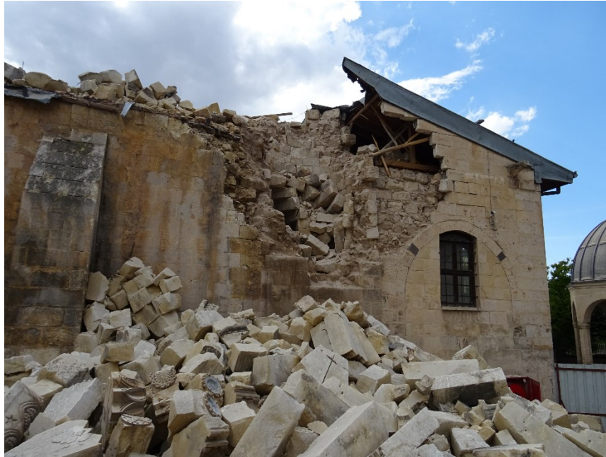
Figure 5.6.34 The mosque after the earthquake, damage due to the collapse of the minaret
