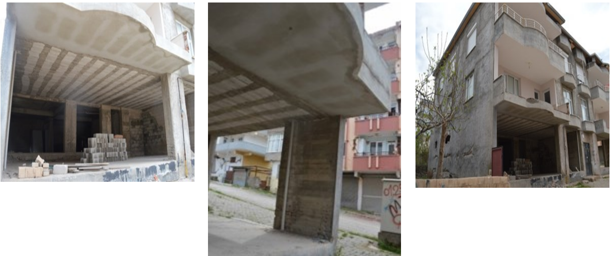
Figure 5.1.22 Building with filler-joist (asmolen) floor system without any apparent damage (Golbasi). Photo: C.Zeris
