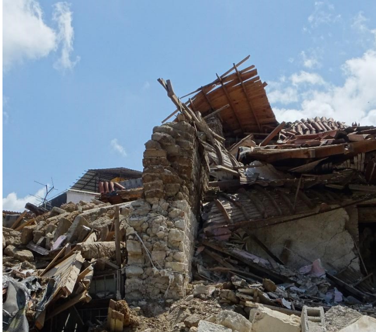
Figure 5.6.11 Antakya, stone masonry (ground floor) and adobe (first storey)
