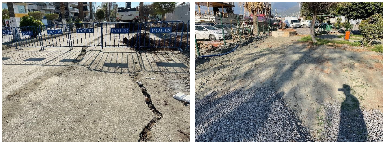
Figure 3.29 (a) Cracks on the road pavement (36.591096N, 36.176768E) and (b) soil ejecta (36.591051N, 36.176851E) because of lateral spreading and soil liquefaction
