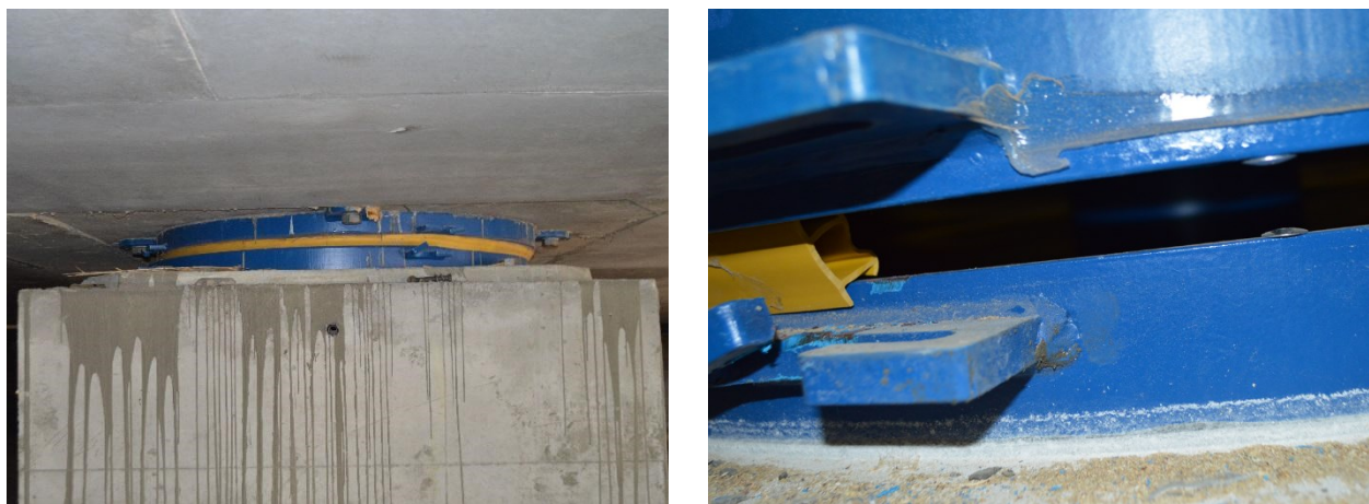
Figure 5.5.4 Kahramanmaraş KDC Hospital (a), (b) broken isolator locks, showing that the isolation system was activated during the earthquake sequence.
