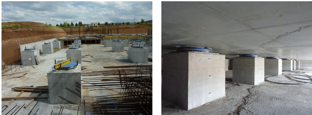
Figure 5.5.3 Kahramanmaraş KDC Hospital (a), (b) bearings layout at the new wings
