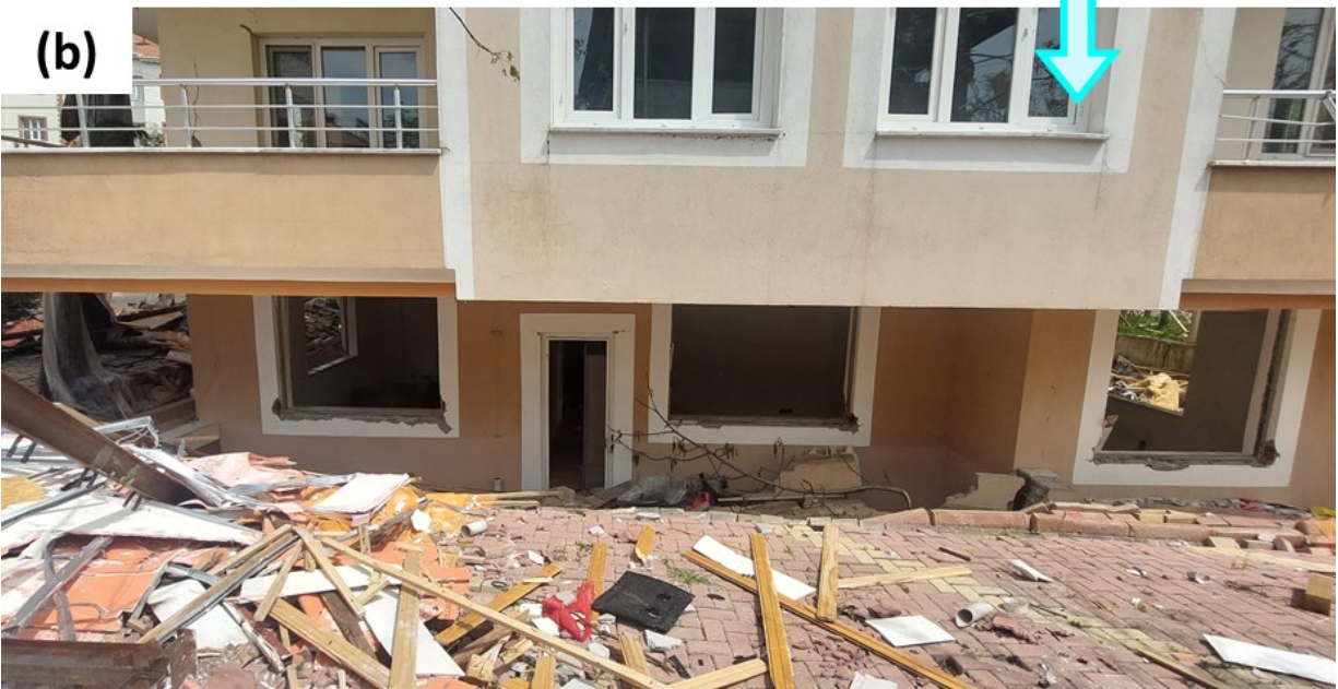
Figure 3.37 (a) Complete and (b) detailed view of a rotated 6-story RC building (37.787913N, 37.646741E)
