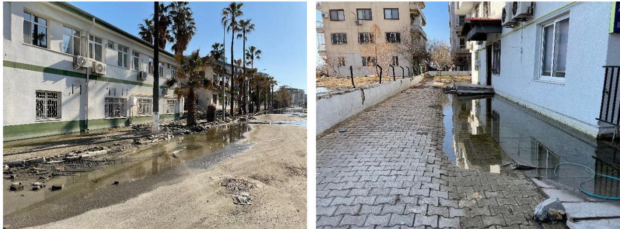
Figure 3.28 Building and pavement subsidence close to the Iskenderun port (a) (36.590425N, 36.179943E) and (b) (36.590425N, 36.179943E)
