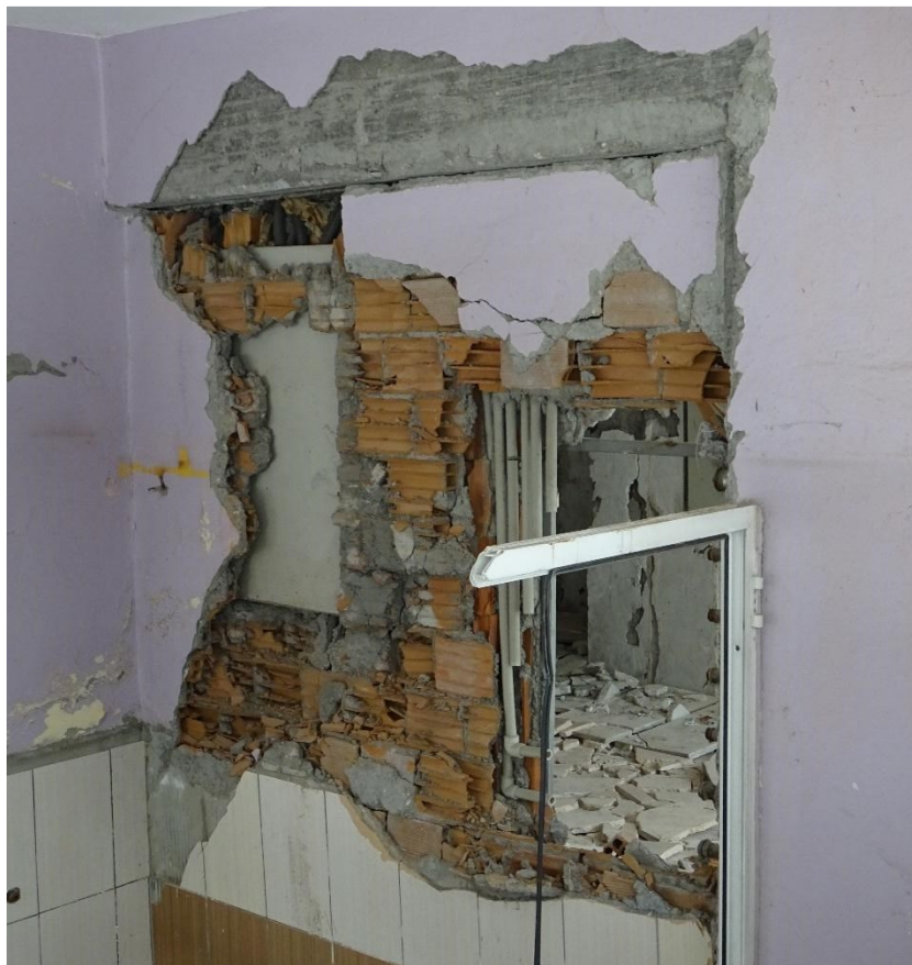
Figure 5.4.6 Carving of the infill walls for installation of electrical and plumbing fixtures.
