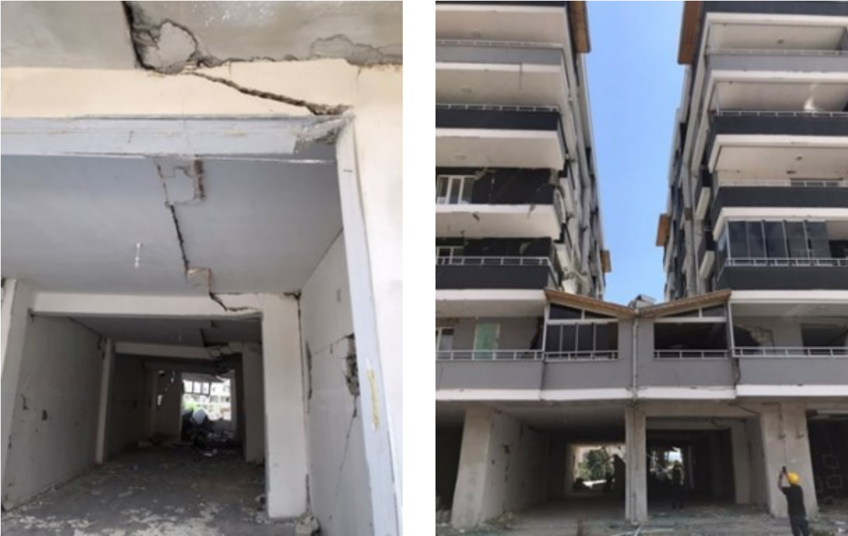
Figure 5.1.19 Inclined cracking in beams caused by non-vertical seismic joint that crosses the beam (Nurdagi). Photo credit: P.Tsopelas
