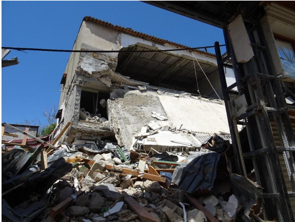
Figure 5.6.26 Antakya, the effect of inadequate intervention using RC slab and jacket to masonry walls.
