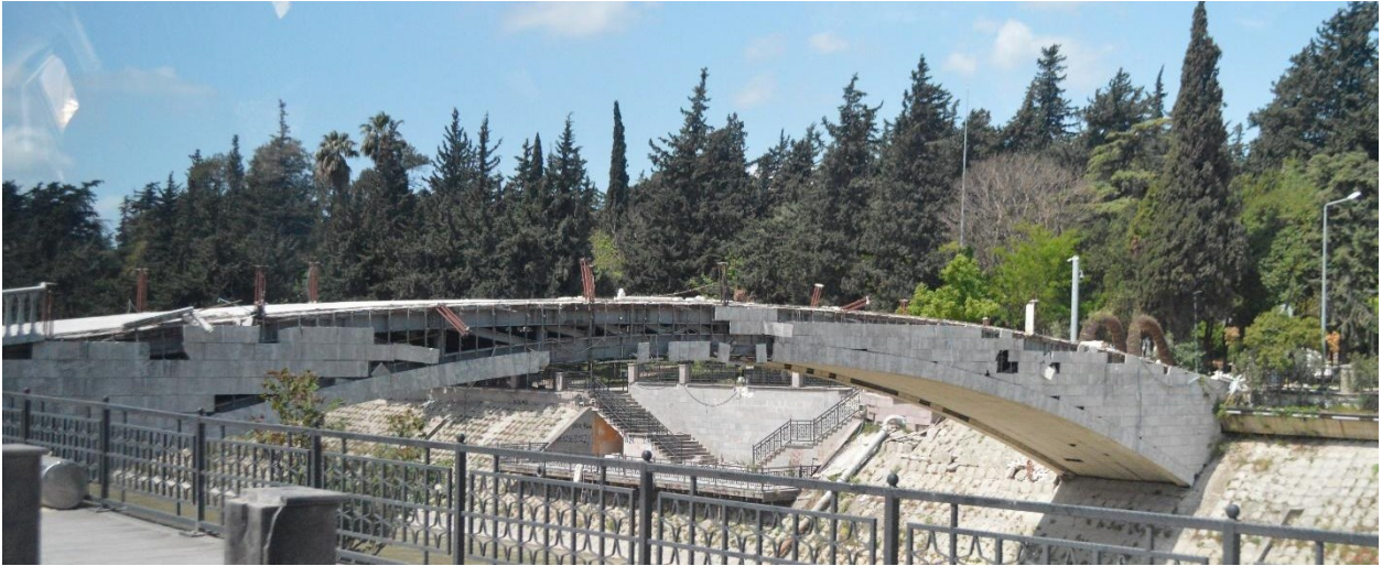
Figure 5.2.13 Steel truss pedestrian bridge with non-structural damage (Antakya).
