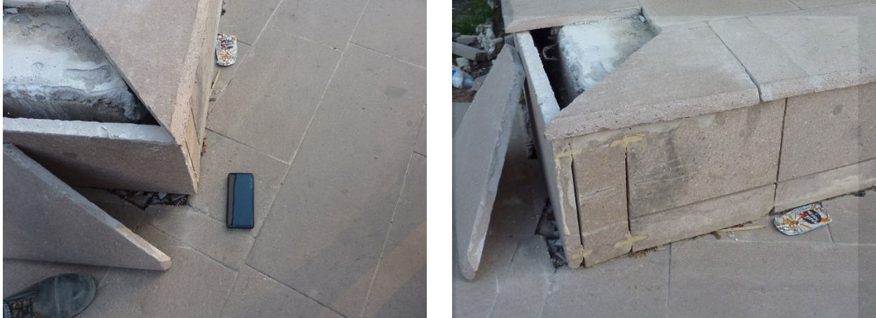
Figure 5.5.8 Dörtyol State Hospital (a), (b) permanent displacement and damaged tiles at the seismic joint
